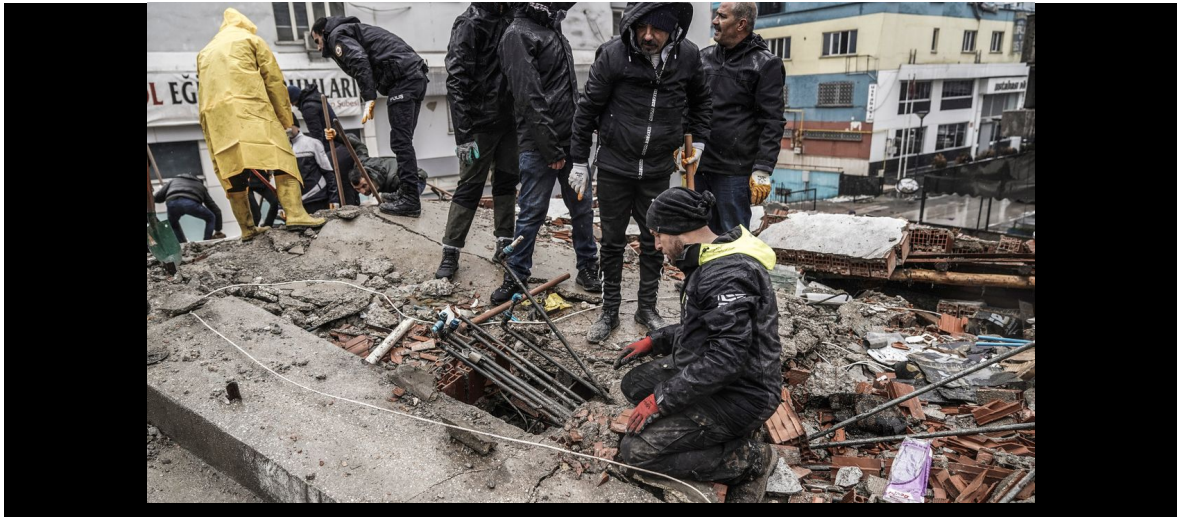
People and emergency teams search for people in the rubble of a destroyed building in Gaziantep, Turkey, Monday, February 6, 2023. [AP Photo/Mustafa Karali]
